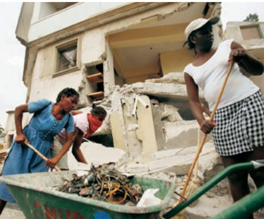
▲ Haitians clean the rubble and debris from the streets as part of a UNDP “cash for work” programme in the Carrefour Feuille of Port-au-Prince.
